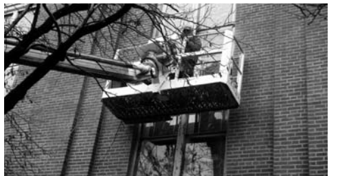
Workers from Rallo Co. applying over 1500 ft. of new trim boards around the 15 stained glass windows.
